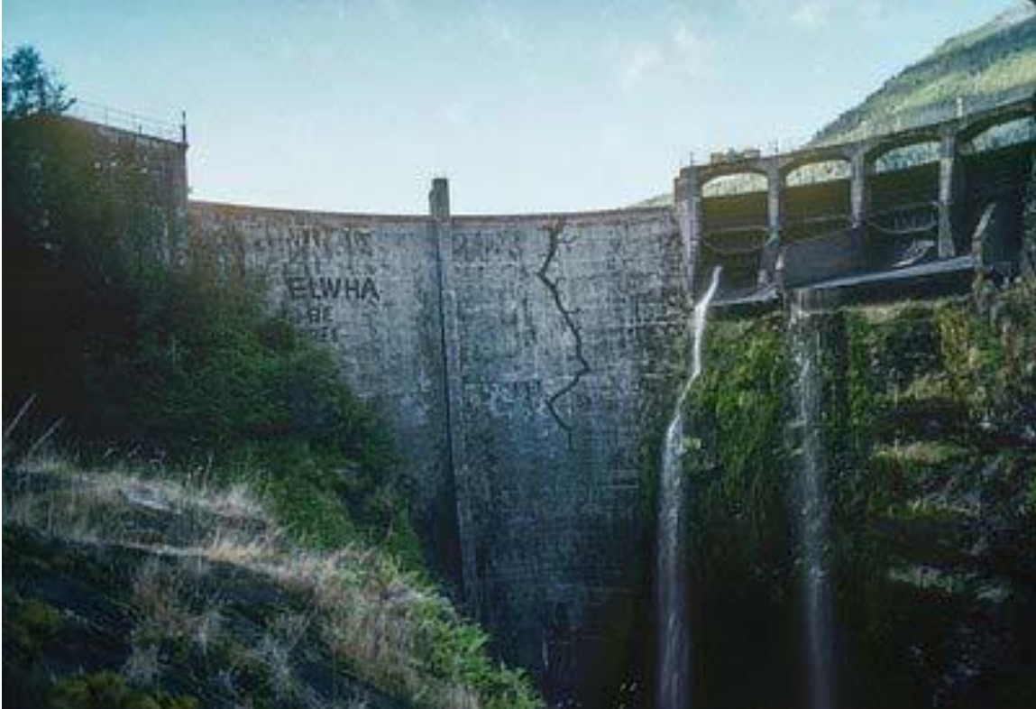
Figure 2: “Elwha Be Free” and painted crack. 1987. Photo courtesy Mikal Jakubal.
